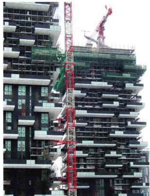
Two residential towers, 80 and 112 m high under construction in February 2013. Large trees and shrubs have already been planted on the lower floors. Bushes and ground-cover plants will also be planted. © König
