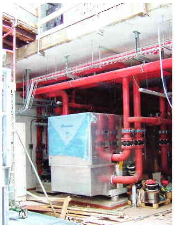
One of the 4 pumps in the underground technology centre. Geothermal energy from groundwater is used to provide warm water. © König
